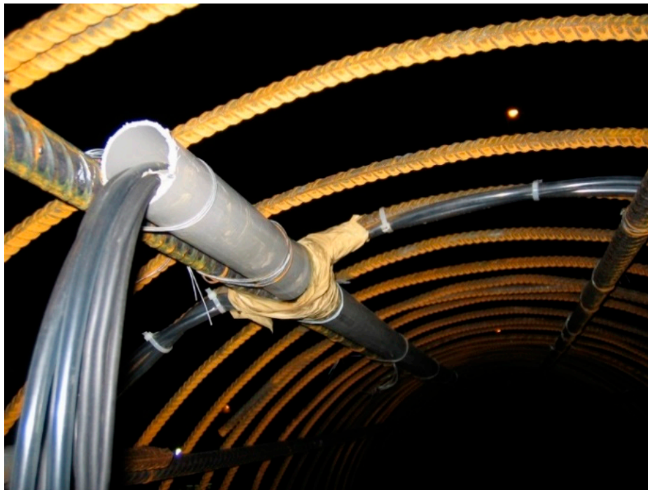
Figure 8. The electrical lead wires from the sensors come to the top.
